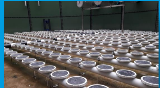
Moving Bed Biofilm Reactor at Lower Gornal
