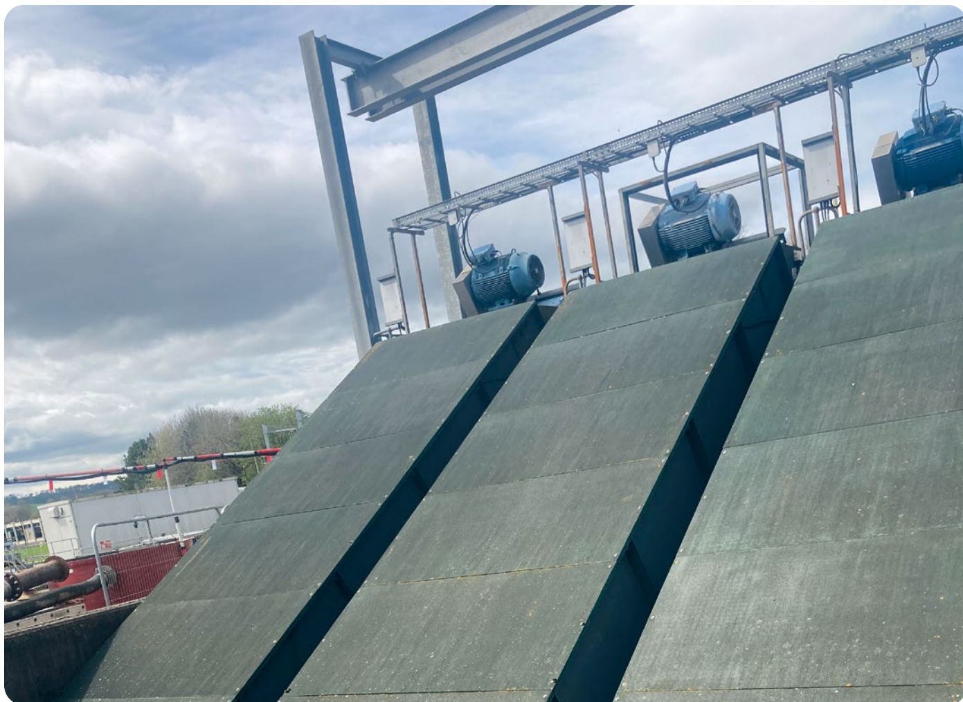
Screw pumps at Barlaston
